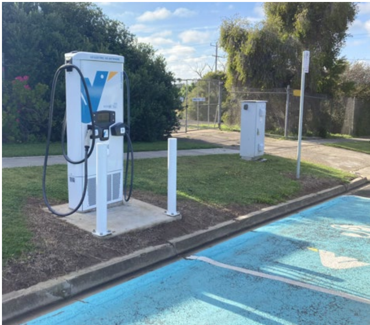
Electric Vehicle Charging Station – Edenhope
